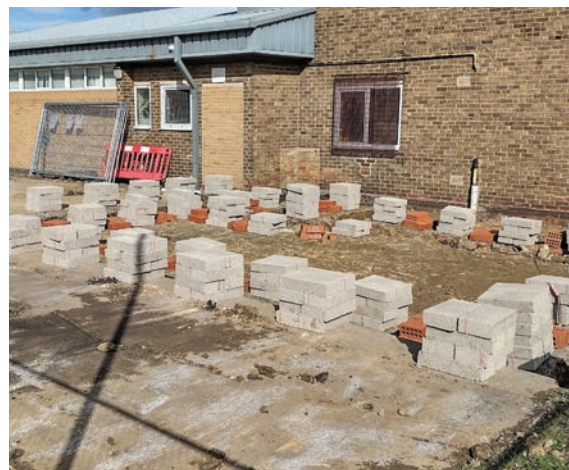
Over a dozen insulation sheets were stolen from the site of the new extension, which will be used to house the many donations made to Woodhouse Close Church foodbank.
