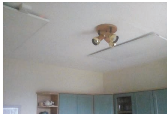
Far infrared panels installed on the ceiling.
